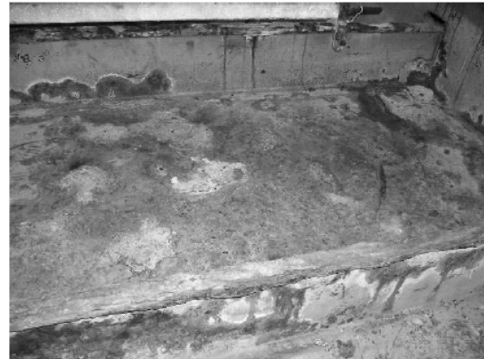
Fig 1 Ship's structural damage due to corrosion
